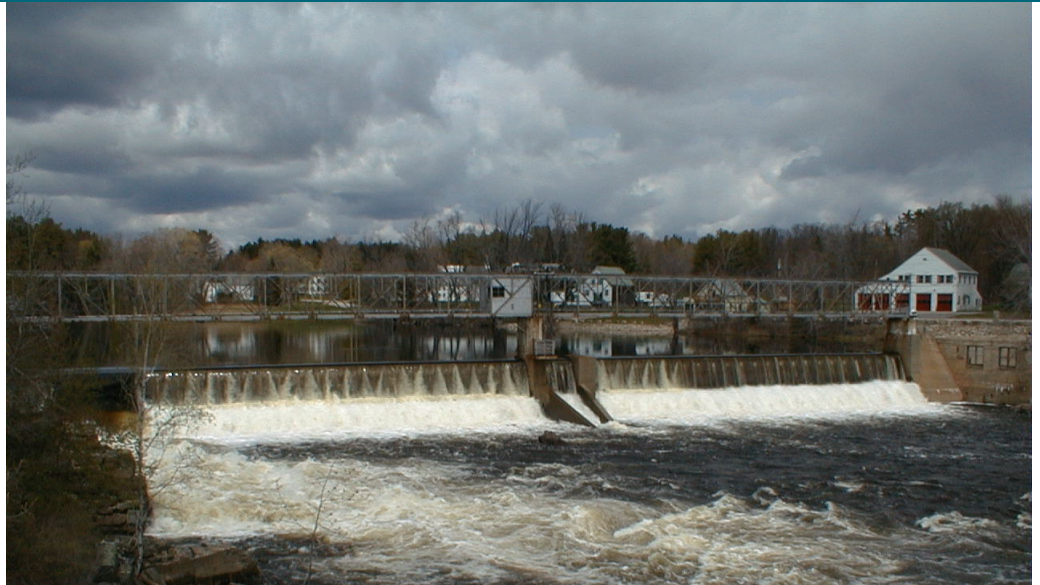
New fish passages to be installed at Bar Mills Dam on Saco River in Maine (credit: Lary Miller, USFWS)
